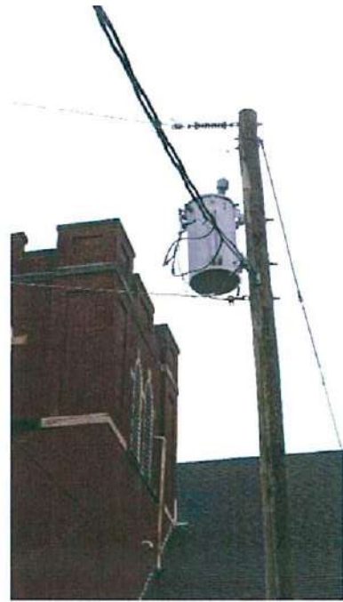
Photo E2 Utility Transformer - outside
