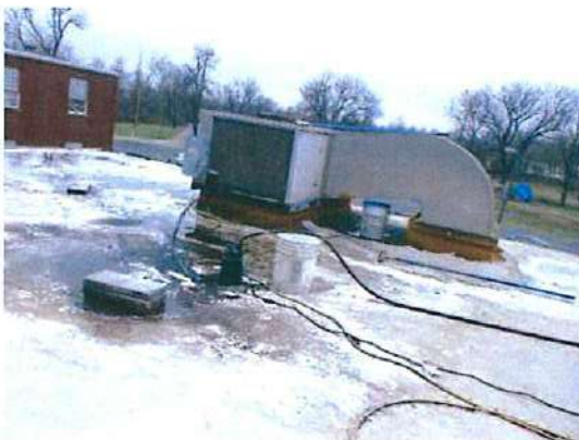
Photo M/P19 Typical Rooftop Unit and Adjacent Condensate Discharge Condition
