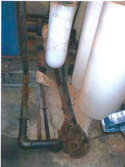
Photo M/P5 Floor Drain Condition
