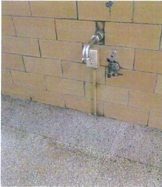
Photo M/P17 Safety Code Violation – Potential Water Contact with Electrical Receptacle
