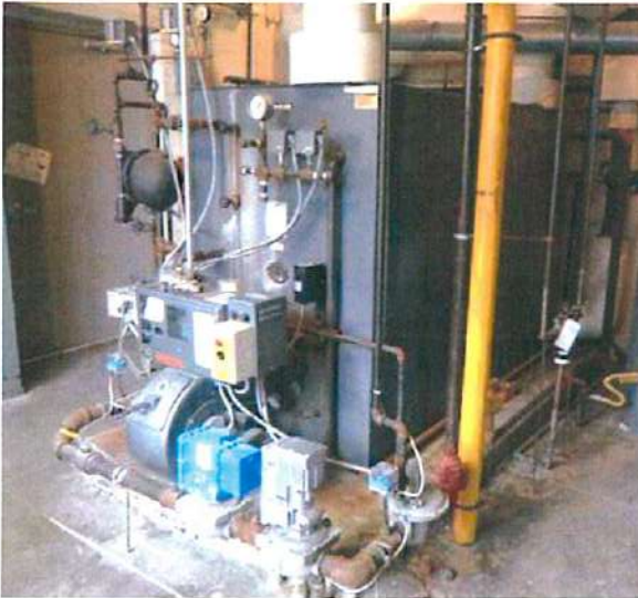
Photo M/P1 Gas-to-Steam Boiler
