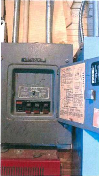
Photo E5 Federal Pacific Load Center – Boiler room
