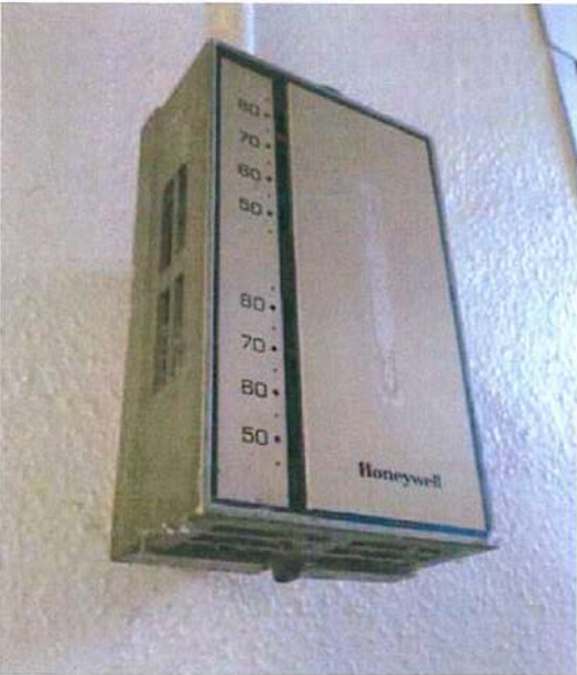
Photo M/P9 Typical Pneumatic Thermostat
