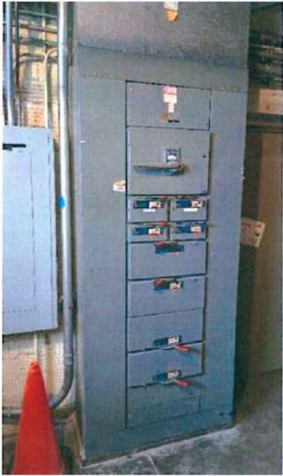
Photo E1 Main Distribution Panelboard (MDP) – Boiler Room
