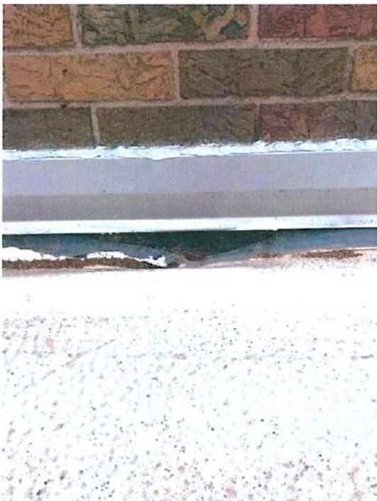
Photo A18 Roof – Membrane not attached properly
