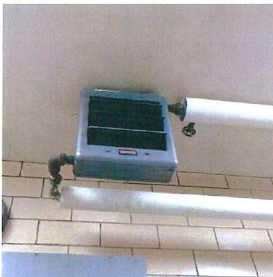
Photo M/P7 Typical Steam Unit Heater
