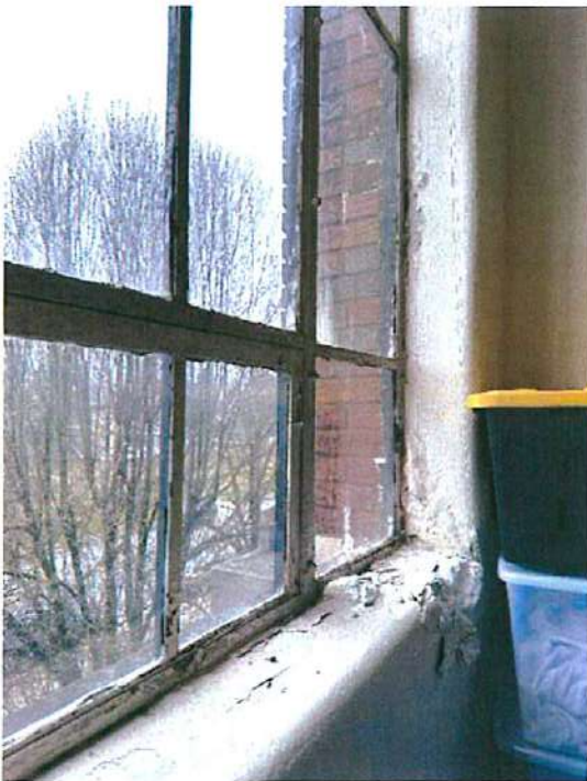
Photo A15 Third Floor – Damage from water intrusion at window
