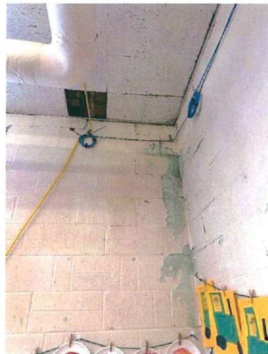
Photo A4 First Floor – Damage to paint due to water seepage at exterior walls
