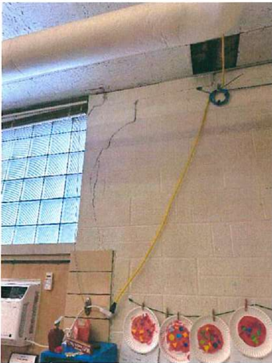
Photo A3 First Floor – Some cracking of exterior wall possibly due to foundation settlement
