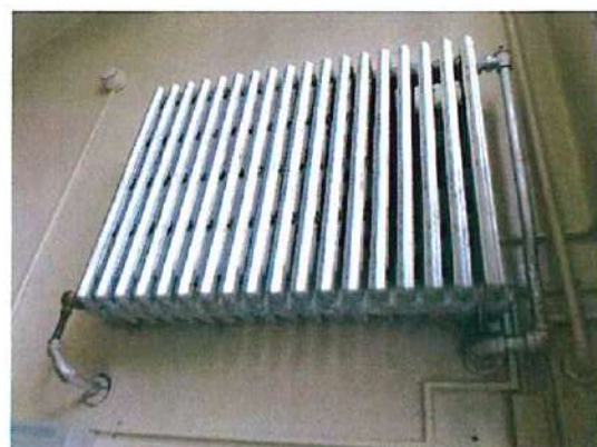
Photo M/P8 Typical Steam Radiant Heating Panel
