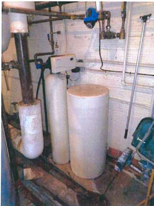
Photo M/P3 Water Softener System
