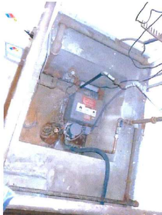
Photo M/P4 Steam Condensate Pump
