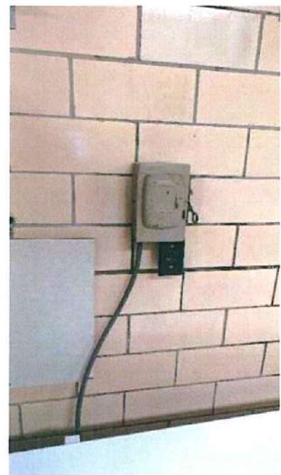
Photo E12 Kitchen Equip DC – Kitchen 114
