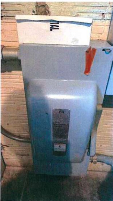
Photo E3 200A Disconnect – Boiler Room
