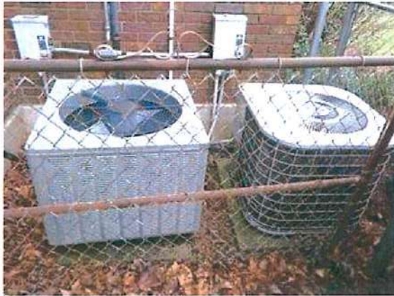
Photo M/P13 Outdoor Heat Pumps
