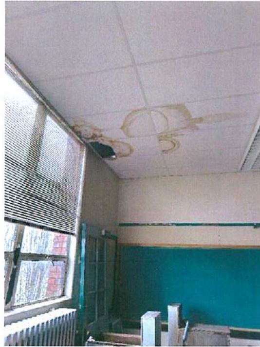
Photo A14 Third Floor – Water damage to ceiling tiles
