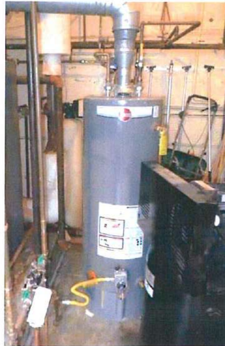
Photo M/P2 Gas Water Heater
