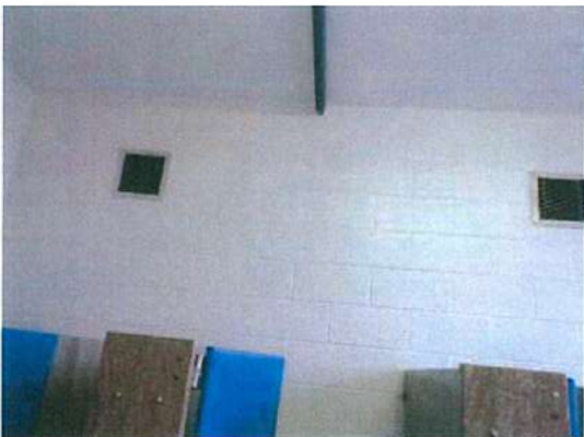
Photo M/P23 Typical Bathroom Exhaust Grille
