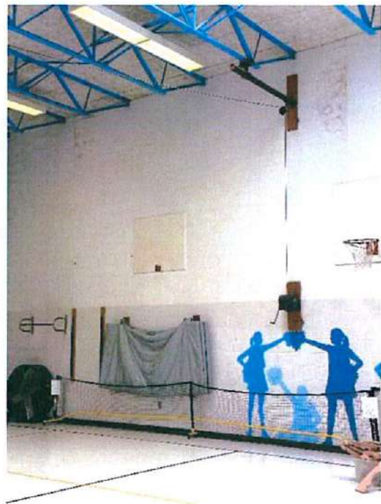
Photo A8 First Floor – Gymnasium; Water damage at some sections of wall
