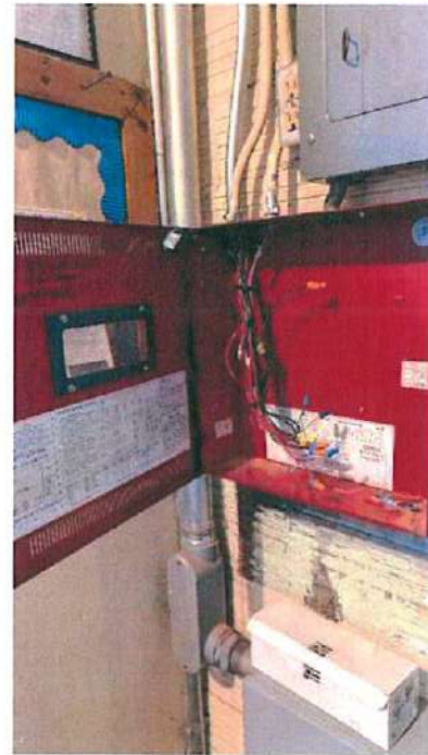
Photo E6 Abandoned FACP – Boiler Room
