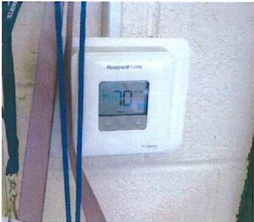
Photo M/P10 Typical Upgraded Programmable Thermostat
