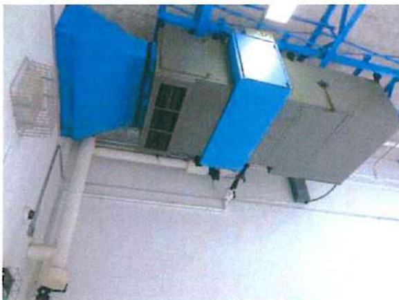
Photo M/P15 Gymnasium – Heating and Ventilating Unit
