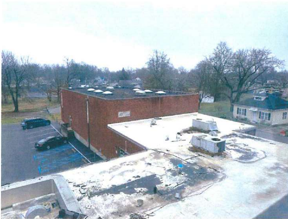
Photo A17 Roof – Standing water on roof
