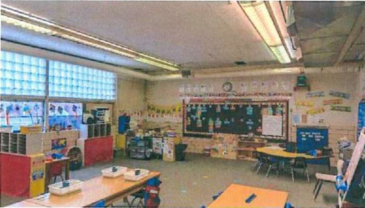
Photo E17 Existing Lighting - Fluorescent
