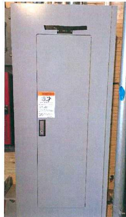
Photo E4 Panel A – Boiler room
