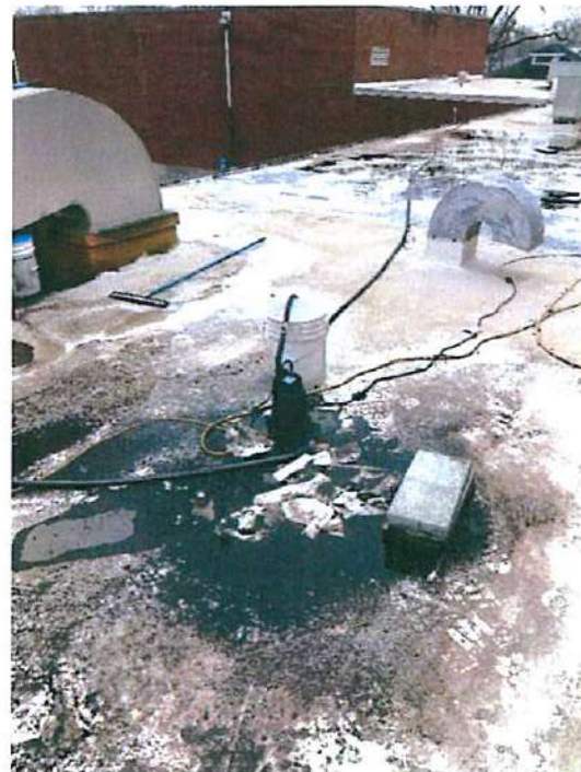
Photo A19 Roof – Sump pumps currently on roof to remove standing water
