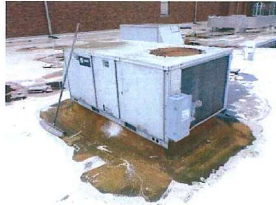
Photo M/P18 Typical Packaged Rooftop Unit
