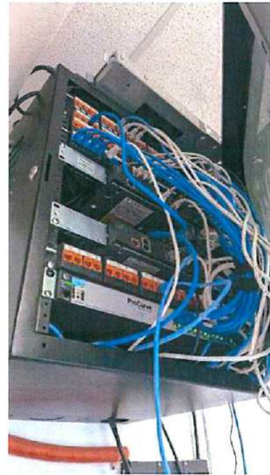
Photo E14 Data Rack – Classroom 110
