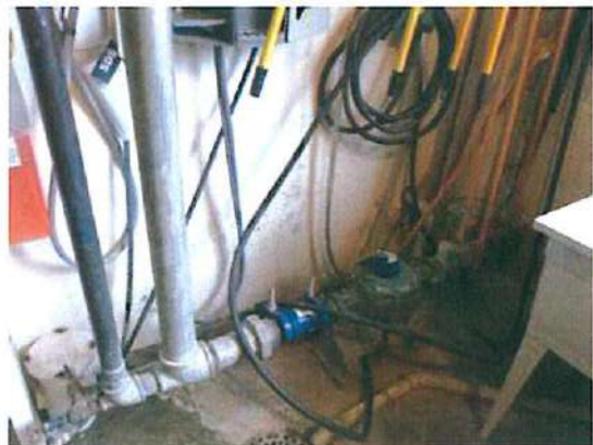
Photo M/P6 Water Entry Service Meter
