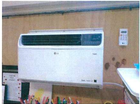
Photo M/P24 Typical Window Air Conditioner
