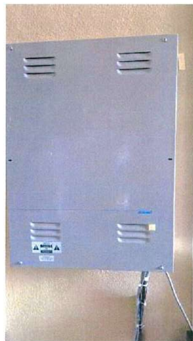
Photo E16 Existing Paging System – Office 203
