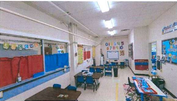
Photo E18 Existing Lighting – LED Retrofit
