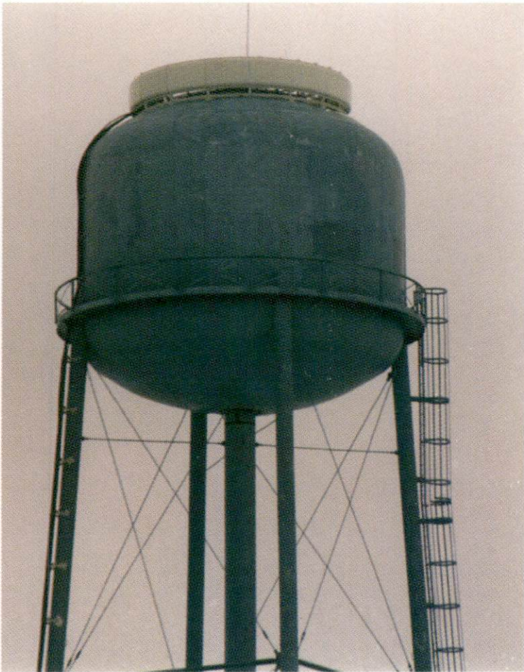
Antenna concealment on already existing Tower
